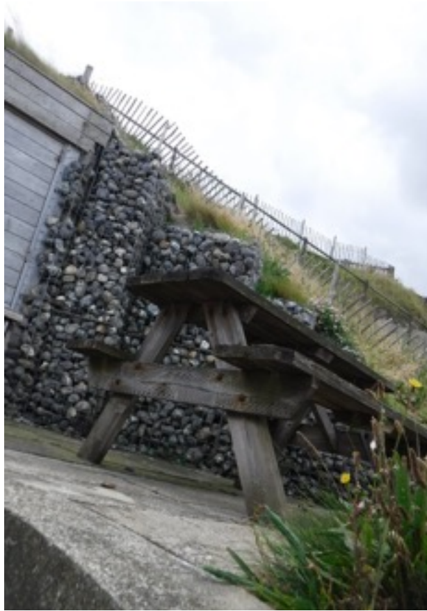
Rock Gabions, Sheringham
