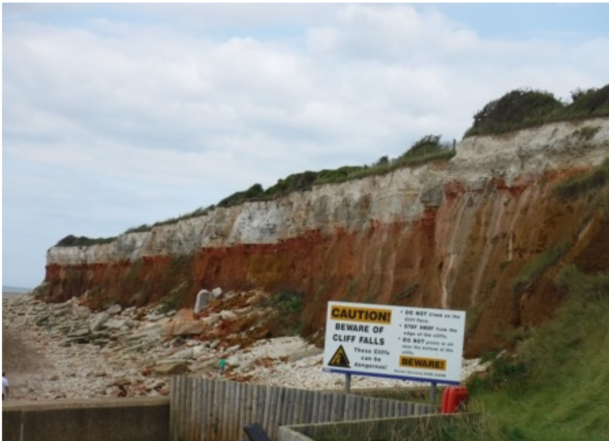
Rubble from unstable cliff face, Hunstanton
