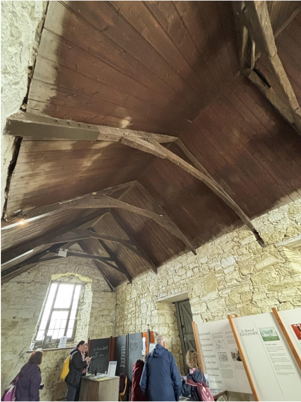
Figure 67: The buildings old roof
